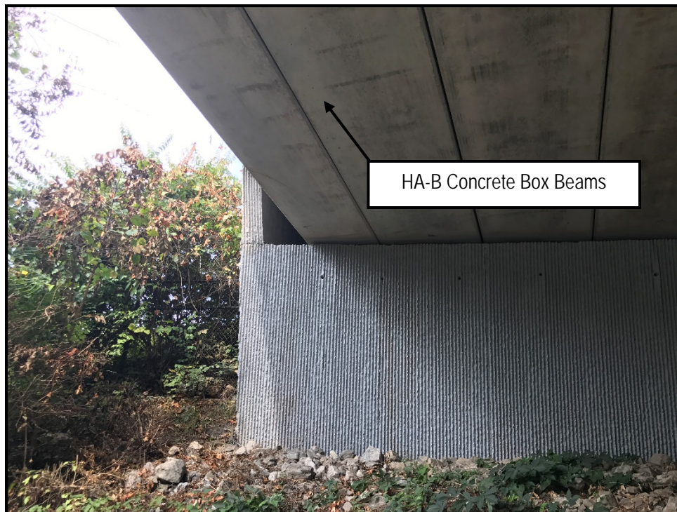
Photo 2: View of HA-B on the eastbound I-440 bridge over Lealand Lane
