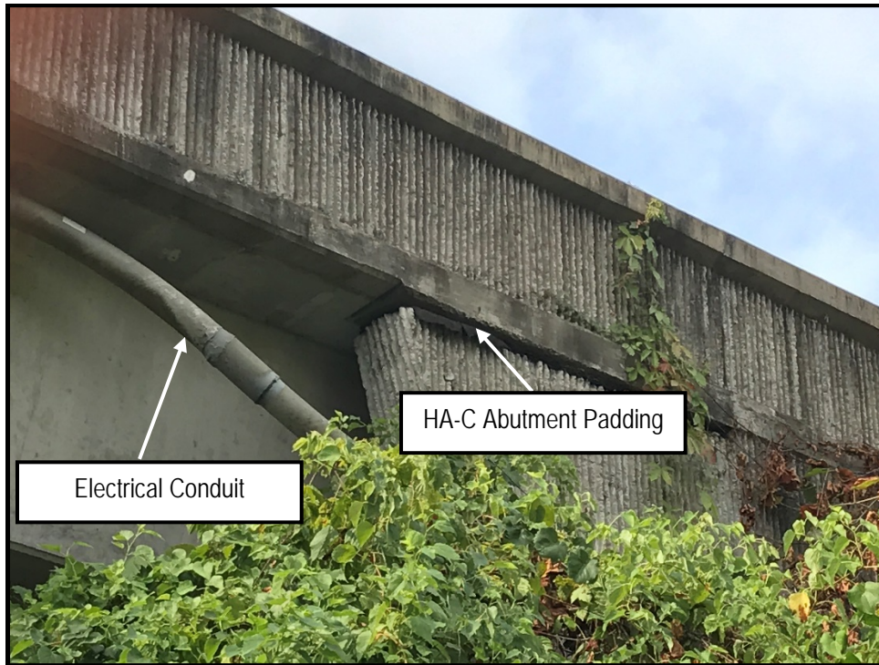
Photo 3: View of HA-C and electrical conduit on the eastbound I-440 bridge over Lealand Lane
