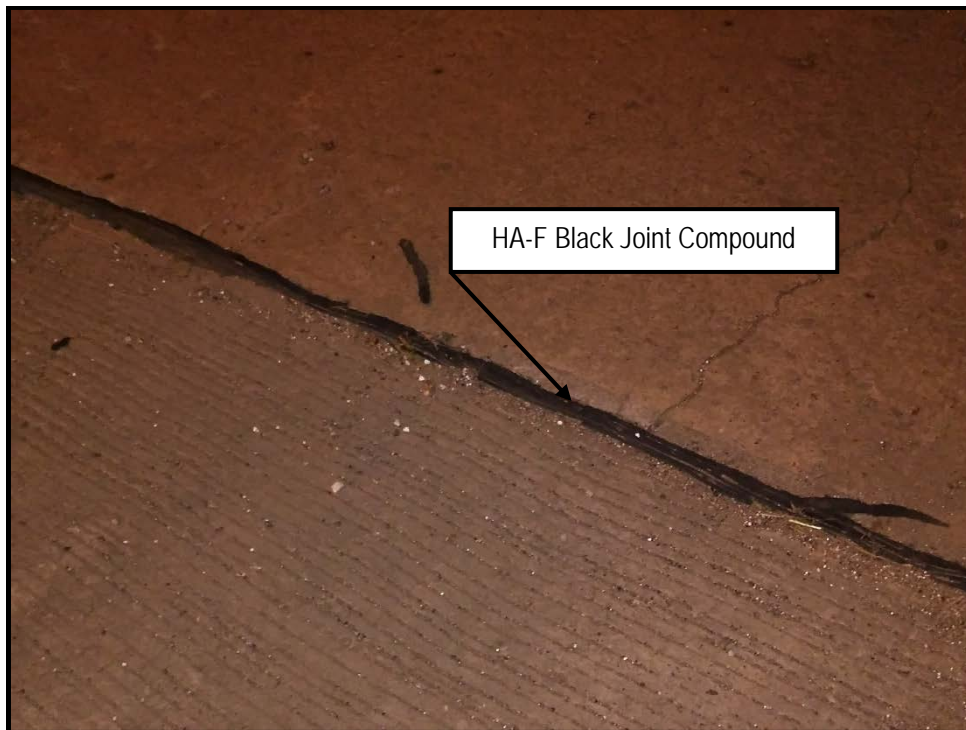
Photo 6: View of HA-F on the eastbound I-440 bridge over Lealand Lane
